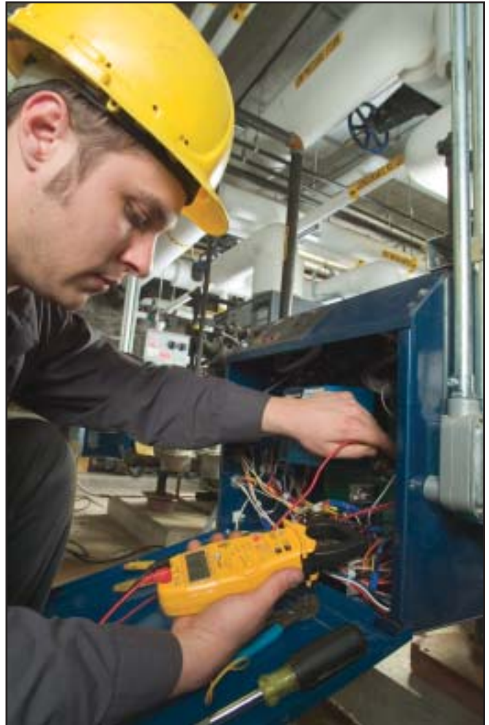
Mike Shilling of Seasonair Inc., Gaithersburg, Md., does control wiring and startup on eight 30-ton computer room systems for a data center in Gaithersburg.
